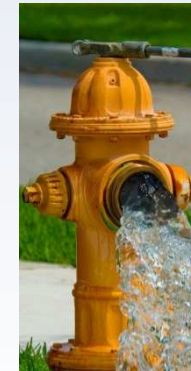
Hydranten (Hose Allowance)
